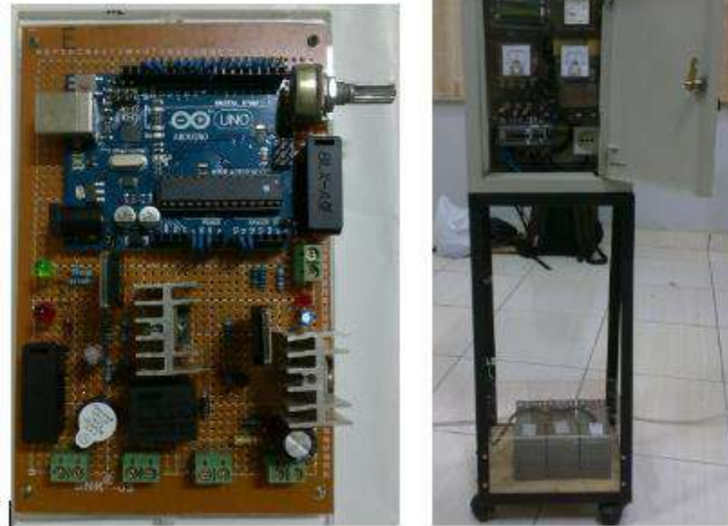
Gambar 10 . Rangkaian Charge Controller
