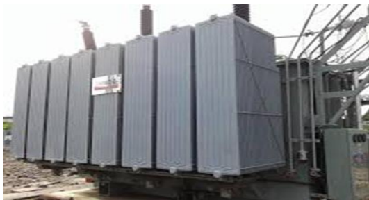
Gambar 4. Transformator Daya 60 MVA UNINDO
