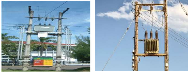
Gambar 1. Transformator jaringan distribusi 20 kv
